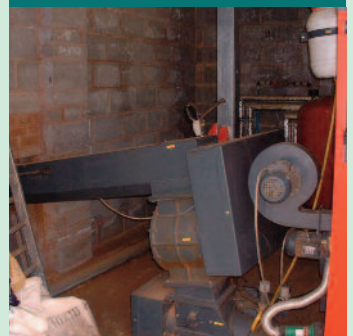
Wood fuel feed to boiler
