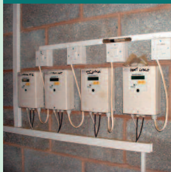
Meters for distributed heat system
