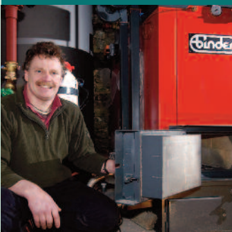
Andy with the boiler
