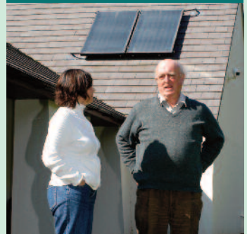
Solar Hot Water panels
