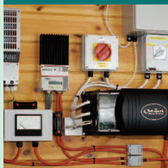
Inverter and charge controllers
