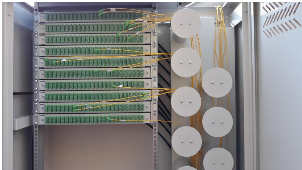
Patch cords leaving the cross-connection cabinet to a cabinet with active devices.
